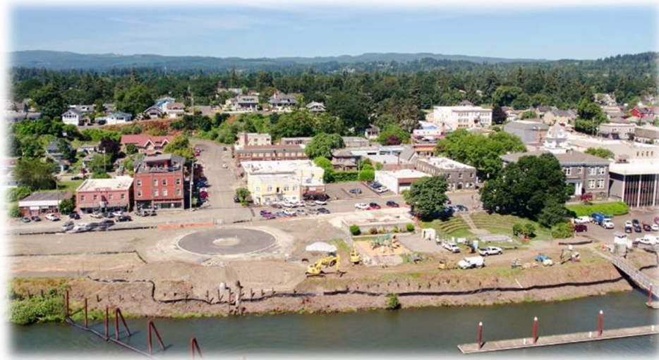
Progress is being made in Columbia View Park as part of the Waterfront Redevelopment Project.
